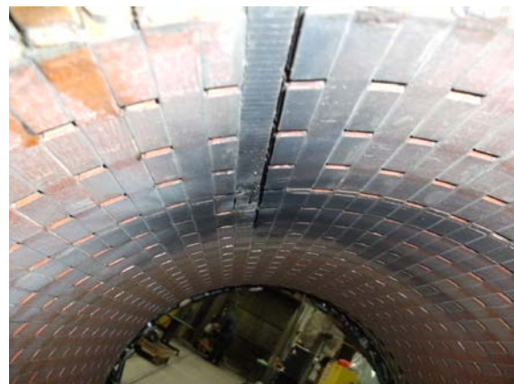
Fig. 1. Failed Stator Coil with Missing Wedge
