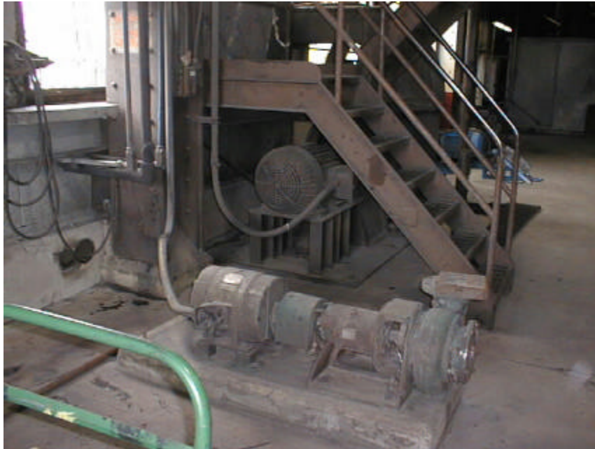
Figure: Pump No Longer In Service
