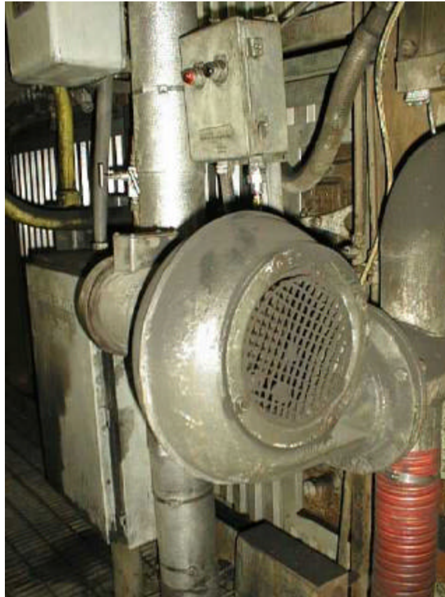
Figure: Dirty Blower
